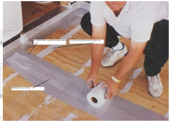
#2 Apply a "pre-stripe" of base coat 5" wide and embed polyester, or fiberglass Tape into the tacky or wet base coat as shown in picture. Alternately, you may use Super Seal Tape to over the crack and pre-stripping is not necessary.
