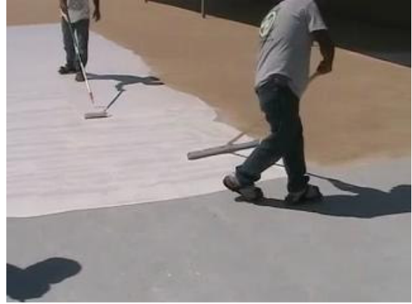
#12 Squeegee and back roll coating. Backroll coating with ½ nap roller. Workman wear spiked shoes for application of coating and back rolling.
