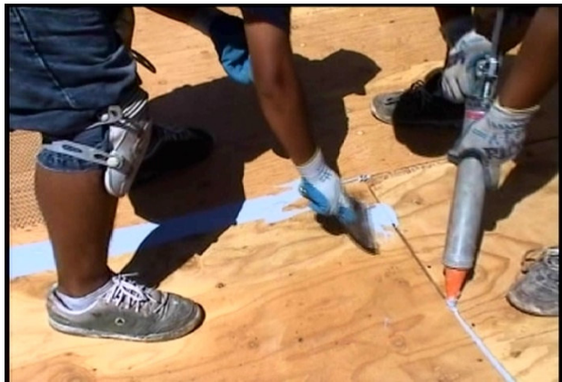
#1 Caulk and Seal with E-101 Sealant all plywood joints. E-101 may be coated over immediately.
