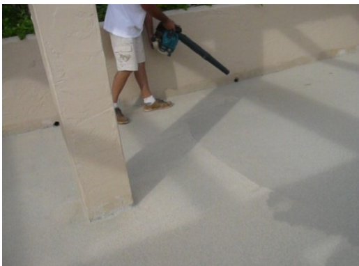
#15 Blow off sand approximately 2 hours for when coating feels completely dry enough to take foot traffic.
