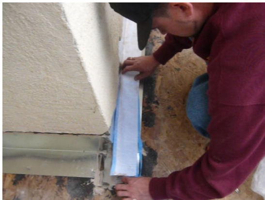
#3 Apply Super Seal Tape to all metal flashings where coating is to be applied. The tape must be completely covered with coating.
