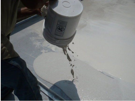
#11 Pour out the coating onto deck and either trowel or squeegee into place. Use notched squeegees to measure out mil thickness.
