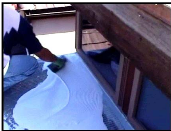
#9 Trowel into place with a 1/8" notch trowel leaving a smooth even surface. Use mil gauge to maintain 50 wet mils on plywood.
