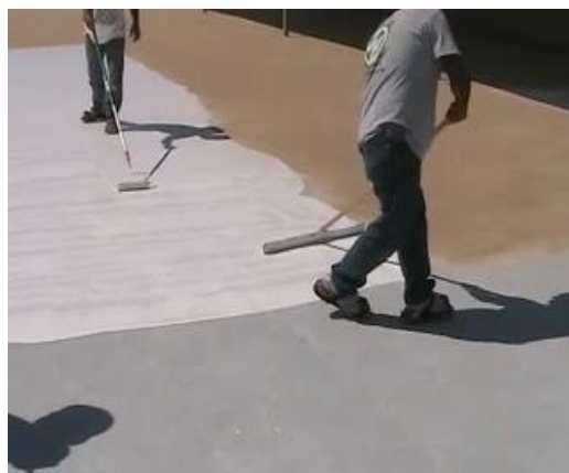
#10 On larger areas, squeegee out the material with a 50 mil notched squeegee and back-roll coating as shown in picture.
