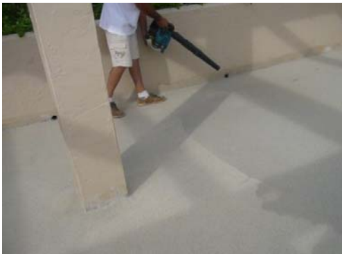
#13 After 3 hours or when coating is walkable without damage, blow and/or sweep all excess sand off the deck.
