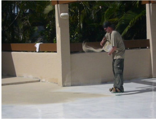
#12 Immediately broadcast 16/30 or 20/40 sand to refusal. Sand should not sink into coating.
